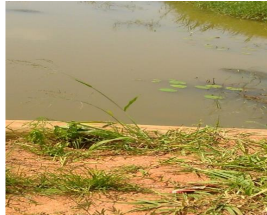
Figure 13: Impact of Reclamation on Infrastructure (Culvert 2018)
