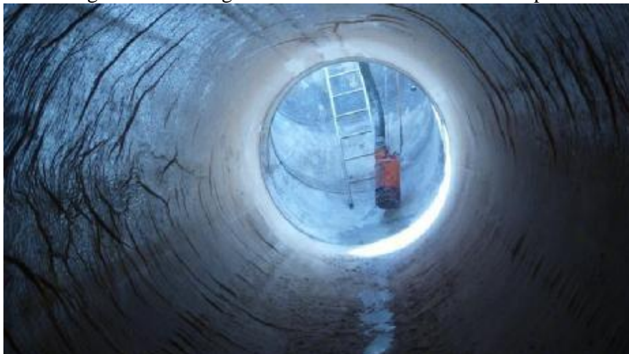
Figure 9: Creasing of Liner on Clarifier 4 Influent Pipe
