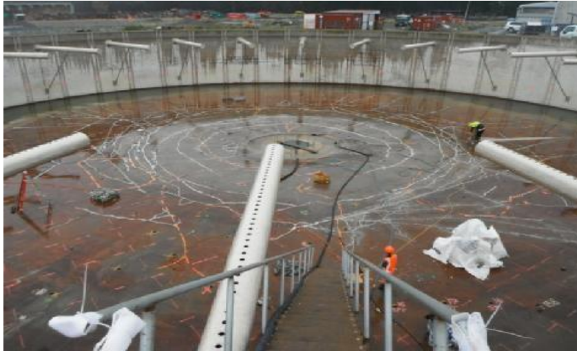
Figure 11: Inverted floor cone on Clarifier 3
