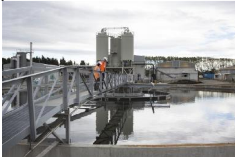
Figure 1: Clarifier 2 at Christchurch Wastewater Treatment Plant
