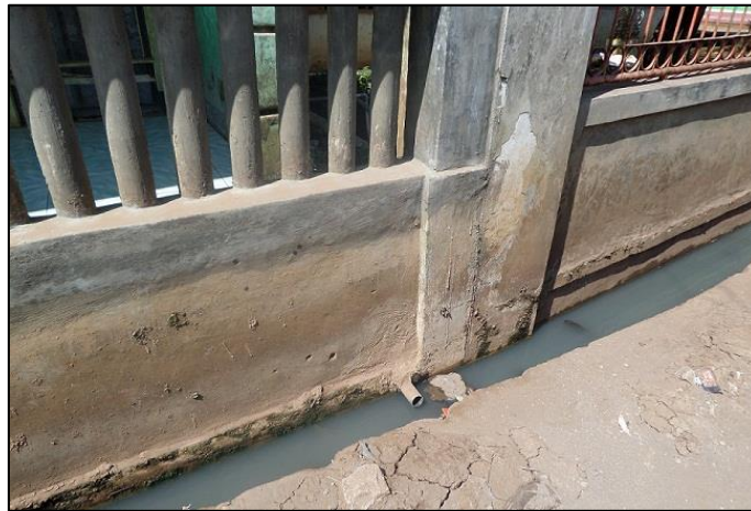
Figure 2.4. Damage Drainage Condition
