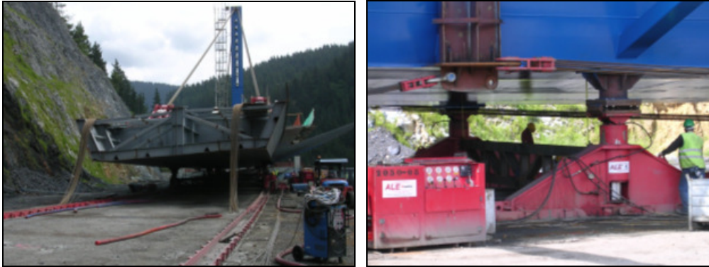
Rear view of the deck during the launching (left) and detailed view of the hydraulic jacks (right)
