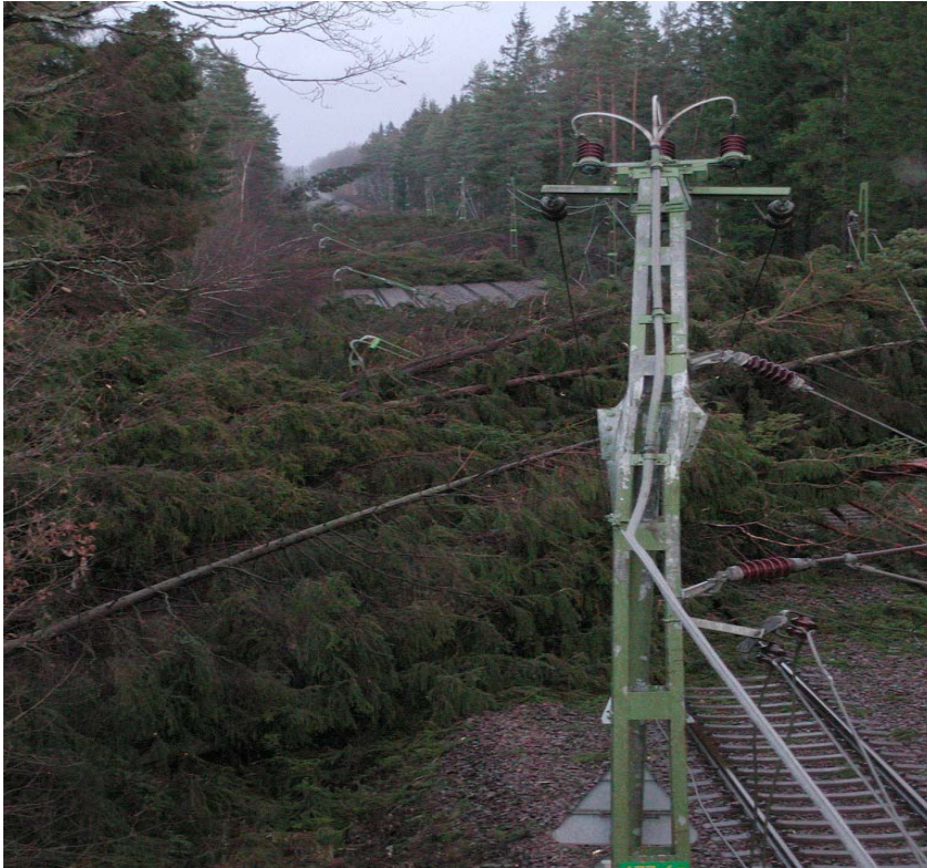
Trees fell across contact wires
