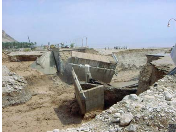
Figure 1. The Arugot Bridge during the May 2001 flood; the bridge collapsed as a result of a headcut backward migration along the stream channel.
