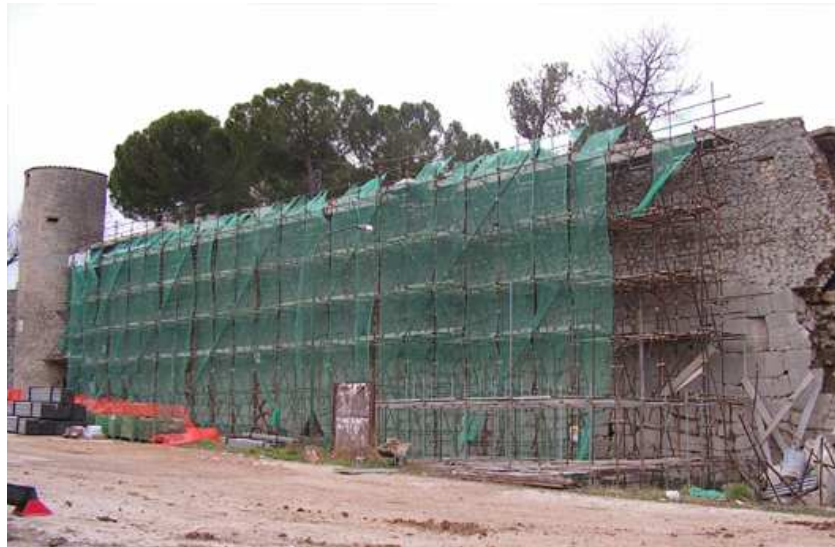
Figure 5 - Partially collapsed wall, presently under restoration
