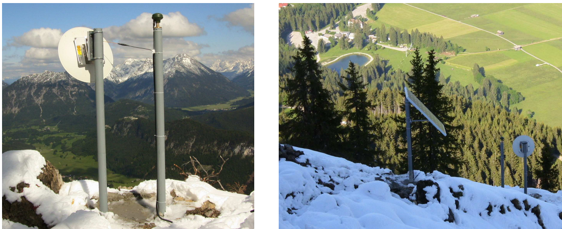
Fig. 10 - Impressions from the Tyrolean Alps near Reutte at an altitude of approx. 1700 m: GNSS sensor nodes equipped with Novatel Smart Antenna, WLAN beam antenna and solar panel.
