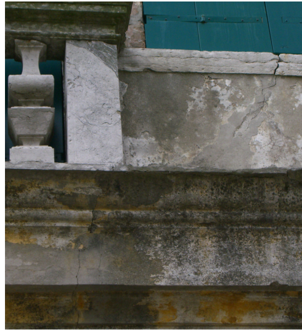
Figure 4: close-up view of the cracking marked by the red circle on the left
