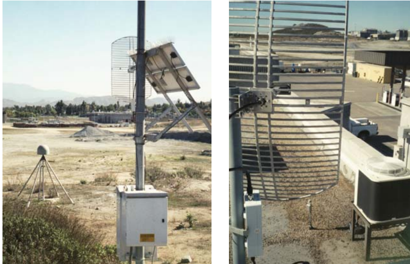
Figure 6. Remote CGPS site with antenna aimed toward backbone site (left) and backbone antenna on roof of building with LAN connection aimed at CGPS site (right).
