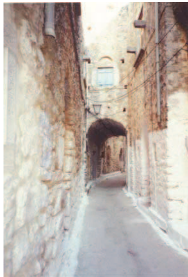
Figure 5: Buildings extending over roads in island settlements (the picture is courtesy of Mrs. M. Fragiskou).
